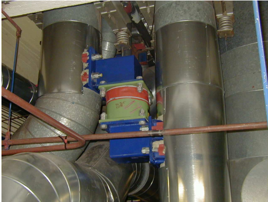
Fig. 10 Connection by VD damper of two RA lines with different dynamic properties.
