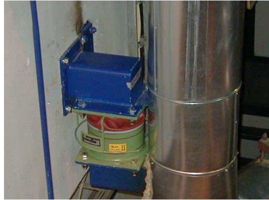
Fig. 11 VRD damper at RA10 line in Turbine Hall (damper's housing at the piping, piston at the wall)
