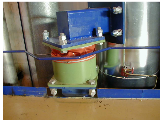
Fig. 9 VD damper at the RA11 in Turbine Hall (damper’s piston at the piping, housing at the TH horizontal floor)
