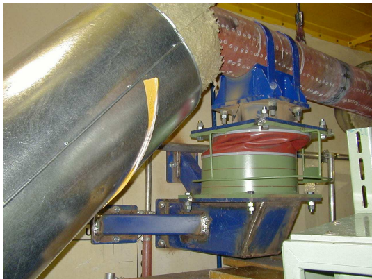
Fig. 8 VES damper at the RL76 in Reactor Building LO2 (damper’s piston at the piping, housing at the RB wall)
