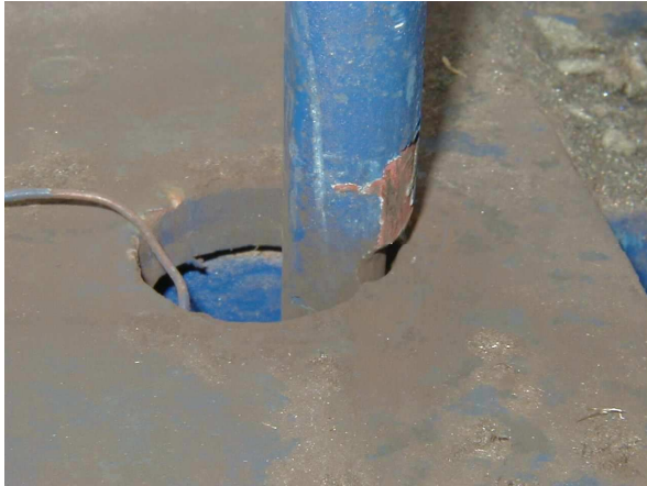
a) wear of the rod hanger
