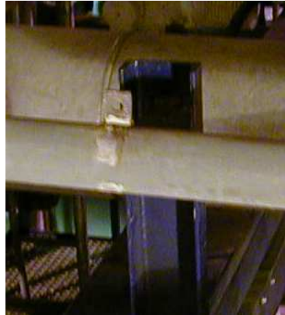
b) fatigue collapse of elastic vibration support
