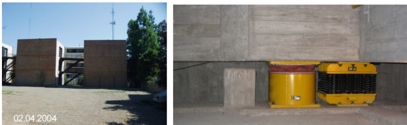
Fig. 13. Two similar structures subjected to earthquake. Isolated by BCS and non-isolated rigid based buildings (left) and location of spring units and viscodampers in the space between sub structure and super structure of the BCS isolated building (right)
