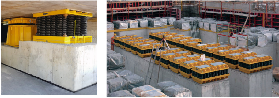
Fig. 3. BCS high capacities spring unit and 3D damper installed between sub and superstructure (left). Installation of the BCS spring units for isolation of multistore building (right).
