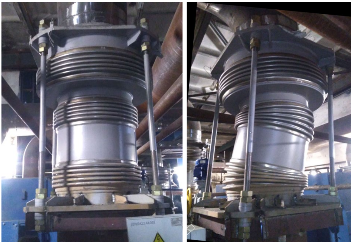
Figure 3. Expansion joint before and after hydrotest
