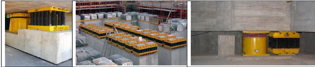
Figure 5. BCS high capacities 3D spring unit and 3D damper installed between sub and superstructure (left, right). Installation of the BCS for the multistore structure (middle), P. Nawrotzki, et. al, (2022).
